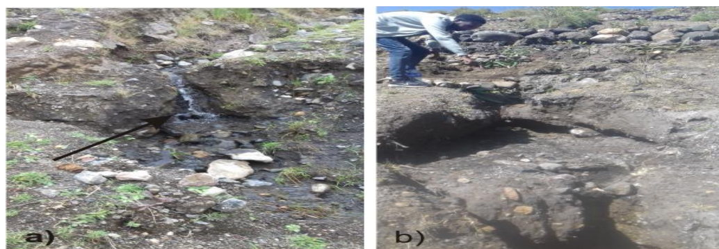
Figure 11. Photographs showing leaking water (a) and erosion features (b) at the downstream face of the embankment. Arrow indicates leaking (flowing) water from the embankment body. Photographs were taken by the second author in 2018.
